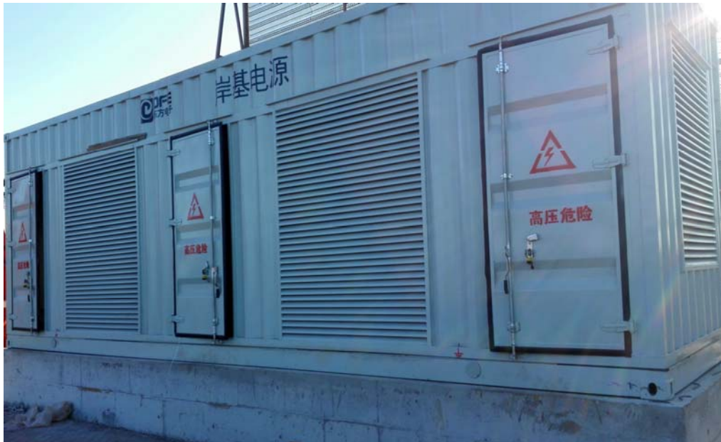
Figure 2 Picture of Variable Frequency Power Supply Equipment
